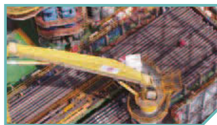
Used UAVs to assist the routing inspection of safety and the screening of hidden dangers
