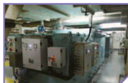
Domestic Sewage Treatment Equipment of Drilling Rig
